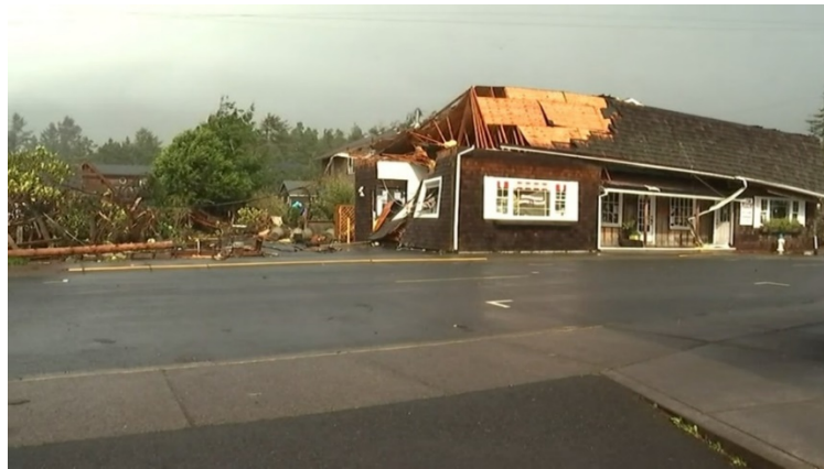
Picture 2-1. Source: KPTV-Manzanita, Oregon tornado damage October 2016
