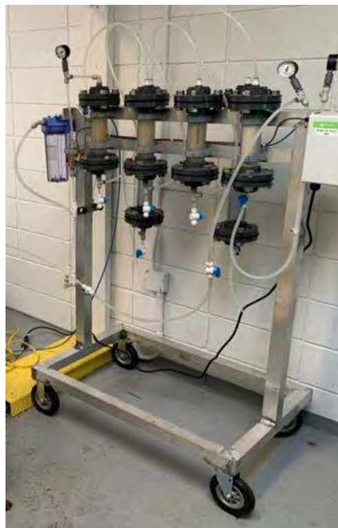
Fig. 2 – Pilot System installed at Chase Well #2
